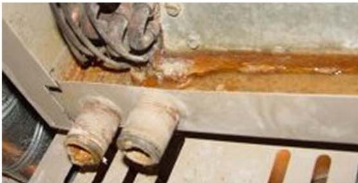
Figure1: Slime problem in drain pan.
